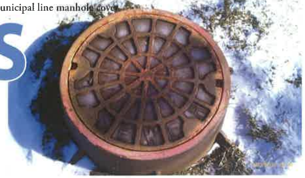
Municipal line manhole cover
